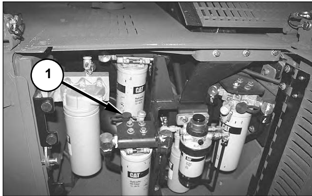
Oil Filter Compartment. (1) Pressure tap (charge pressure).
