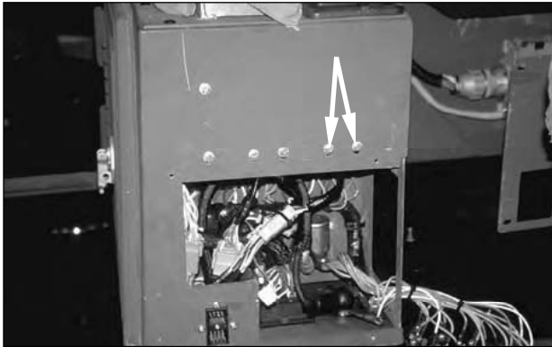
Mounting Location (Arrows) for Number-2 Solenoid Driver-Right Console, Front View, Cover Removed.
