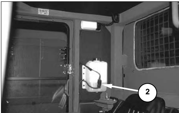
Operator's Compartment, Right Rear Corner. (2) Washer motor.
