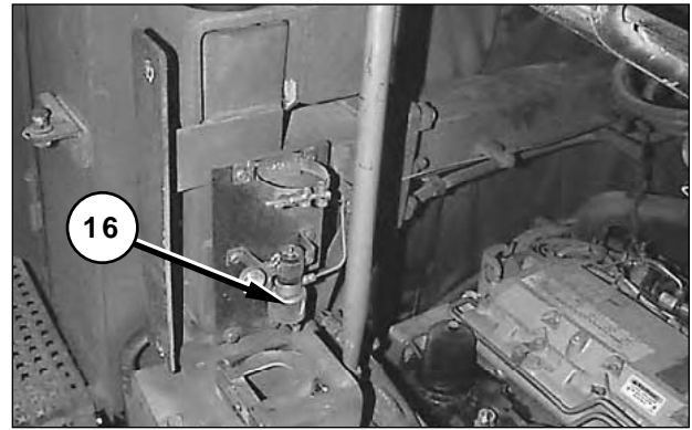
Engine Compartment. (16) Ether injection solenoid.
